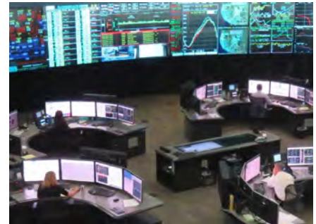
CAISO is preparing for impacts to the grid from public-safety power shut-offs. Photo: Jason Fordney
