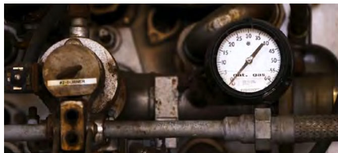
A corroding natural gas pressure sensing line inside Grayson Power Plant reads 0 psig. Photo: Glendale Water & Power
