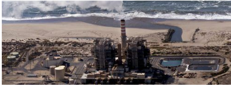
Puente Peaker Plant in Oxnard
