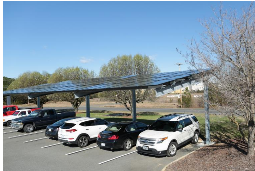
Solar in parking lot as carport
