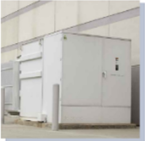
TRANSFORMER ON PAD MATERIAL: METAL COLOR: WHITE
