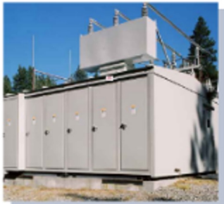
PROJECT MV SWITCHGEAR MATERIAL: METAL COLOR: WHITE
